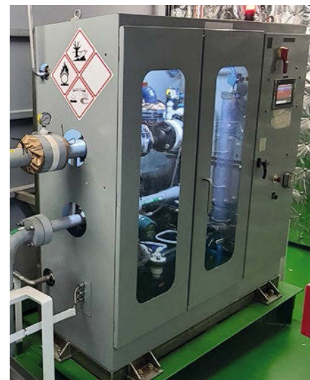
Installed Ecochlor ballast water management system
